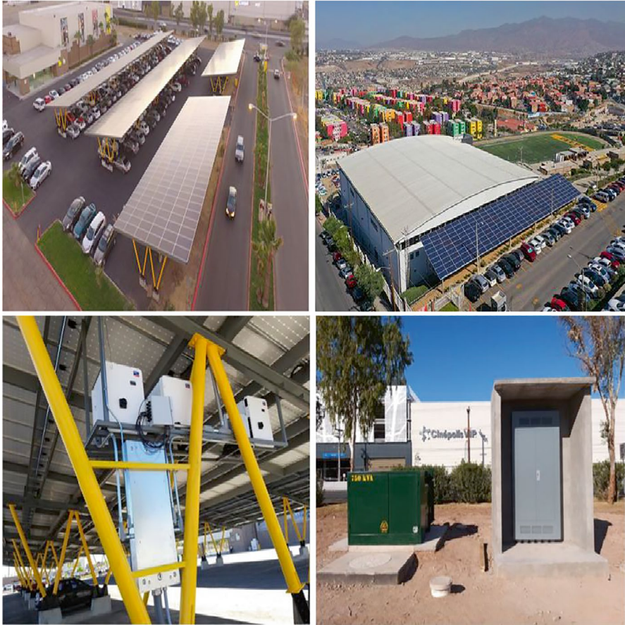
Fig. 4 Photovoltaic generation facilities at CETYS University
